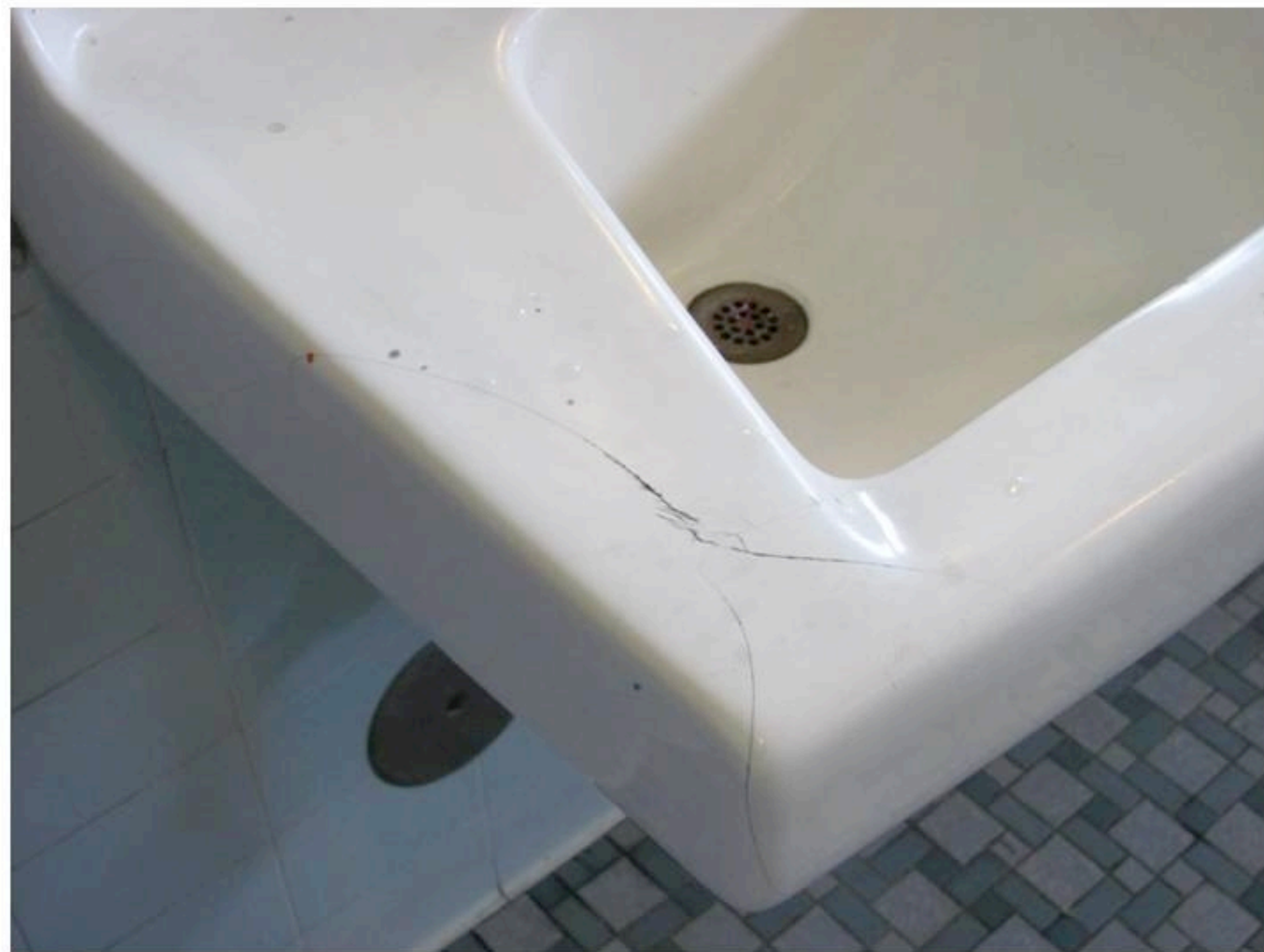
Girls Restroom. Cracked sink.
