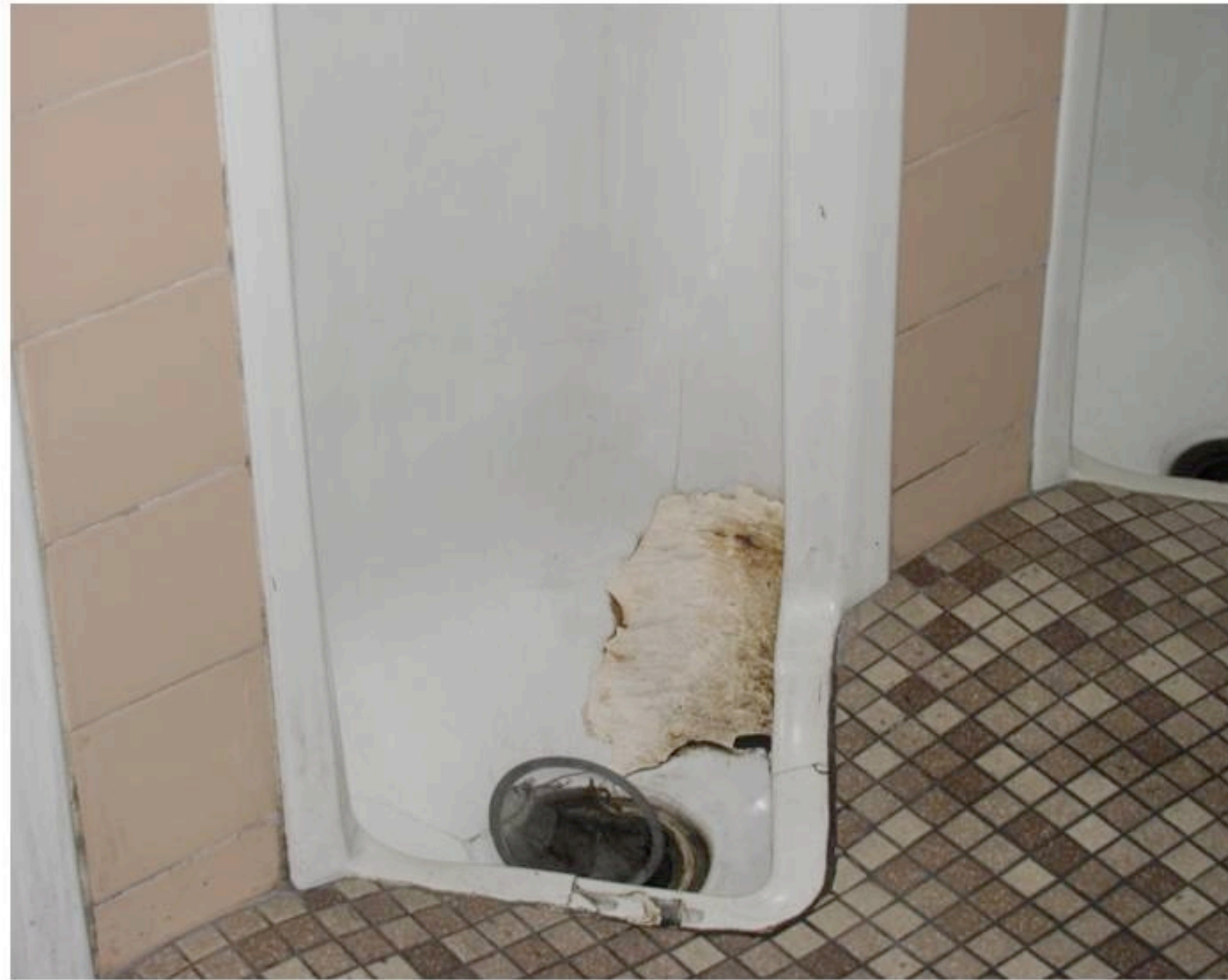
Urinal in Boys Restroom. Deteriorated patch job traps odors and therefore emits a constant unpleasant smell.
